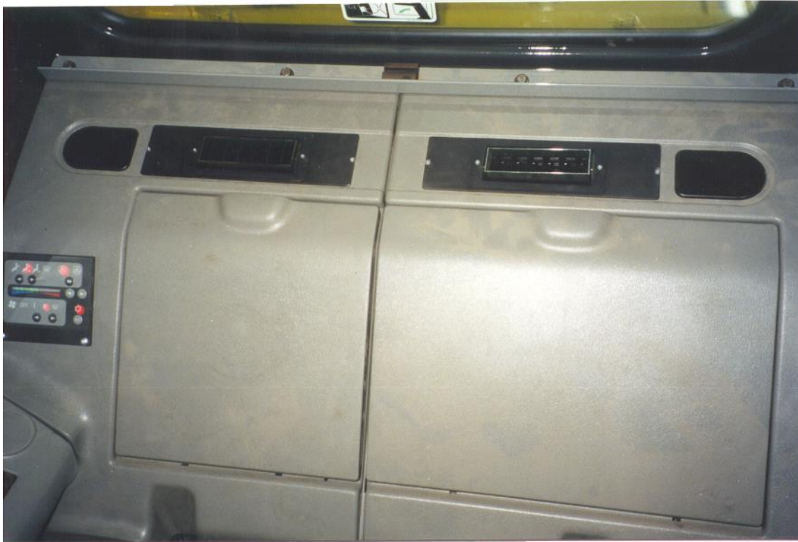
Louvers and controls in place.
